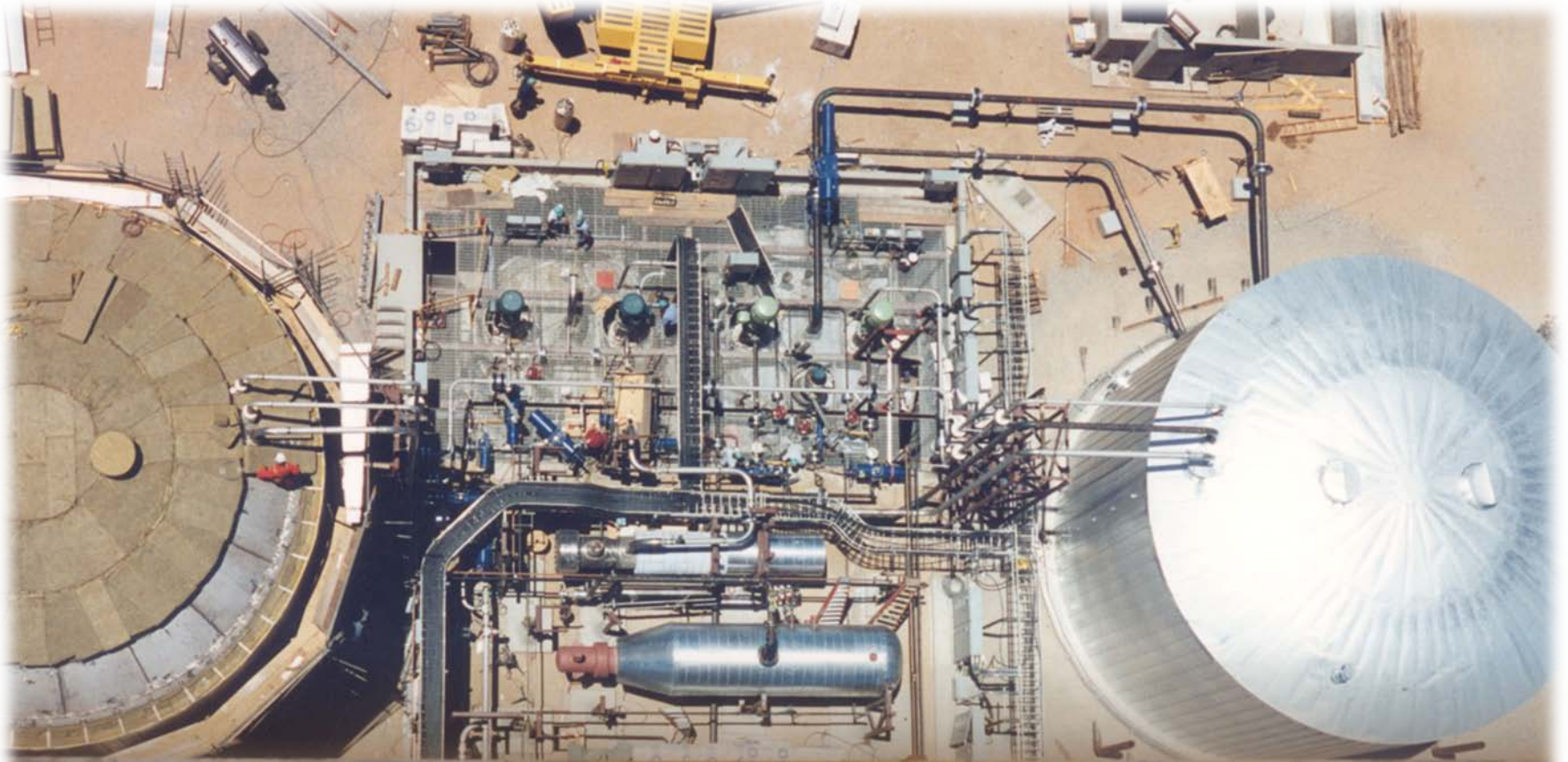
Solar 2 Molten Salt Thermal Storage Tanks and Steam Generators
